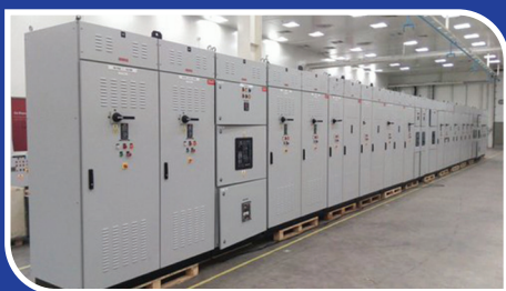
PCC Panel / Switchgear Panel
