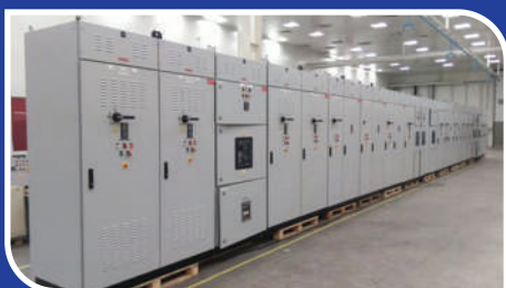
PCC Panel / Switchgear Panel
