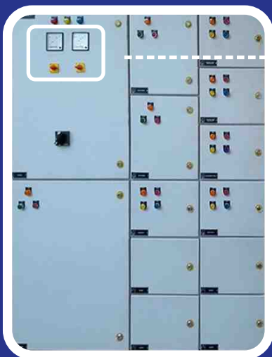
ANALOG VOLTMETER + AMMETERS + 2 NOS. SWITCH
